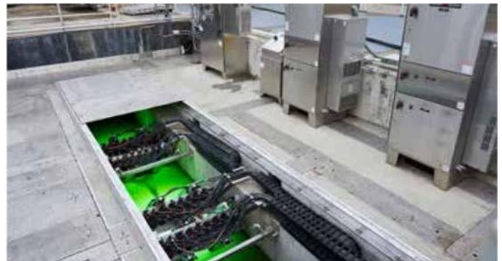
This TrojanUVSigna installation can treat 20 MGD (875 l/s) in only 250 ft 2 (23 m 2 ).
