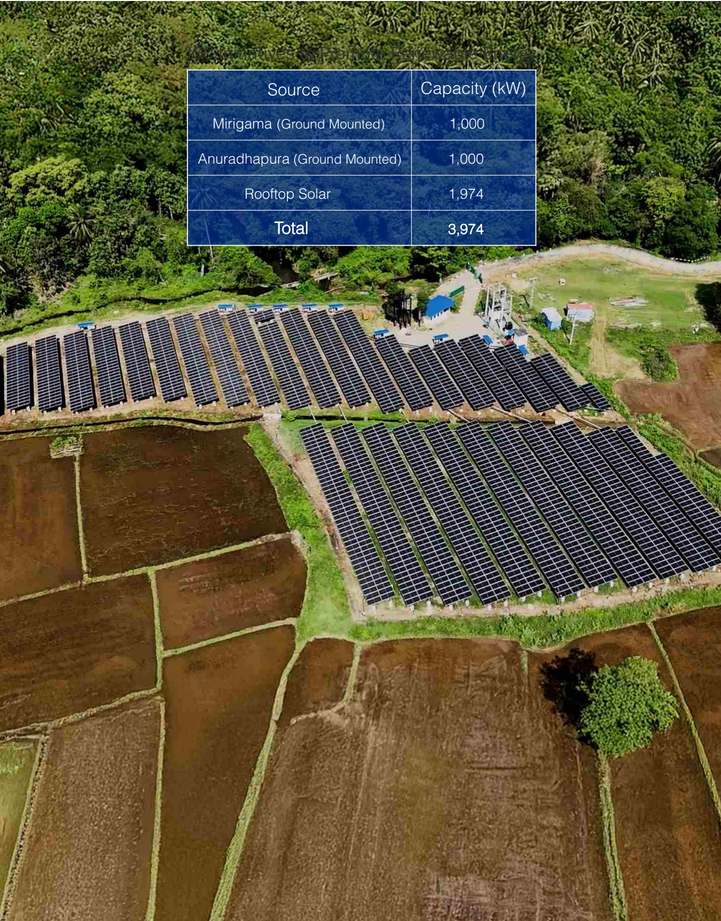
Ground Mounted Solar Power Plant - Thirappane
