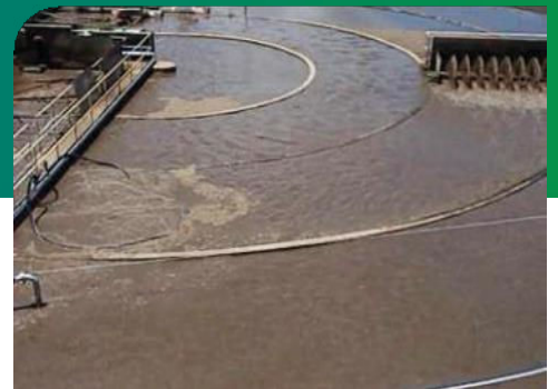
Activated Sludge Systems
